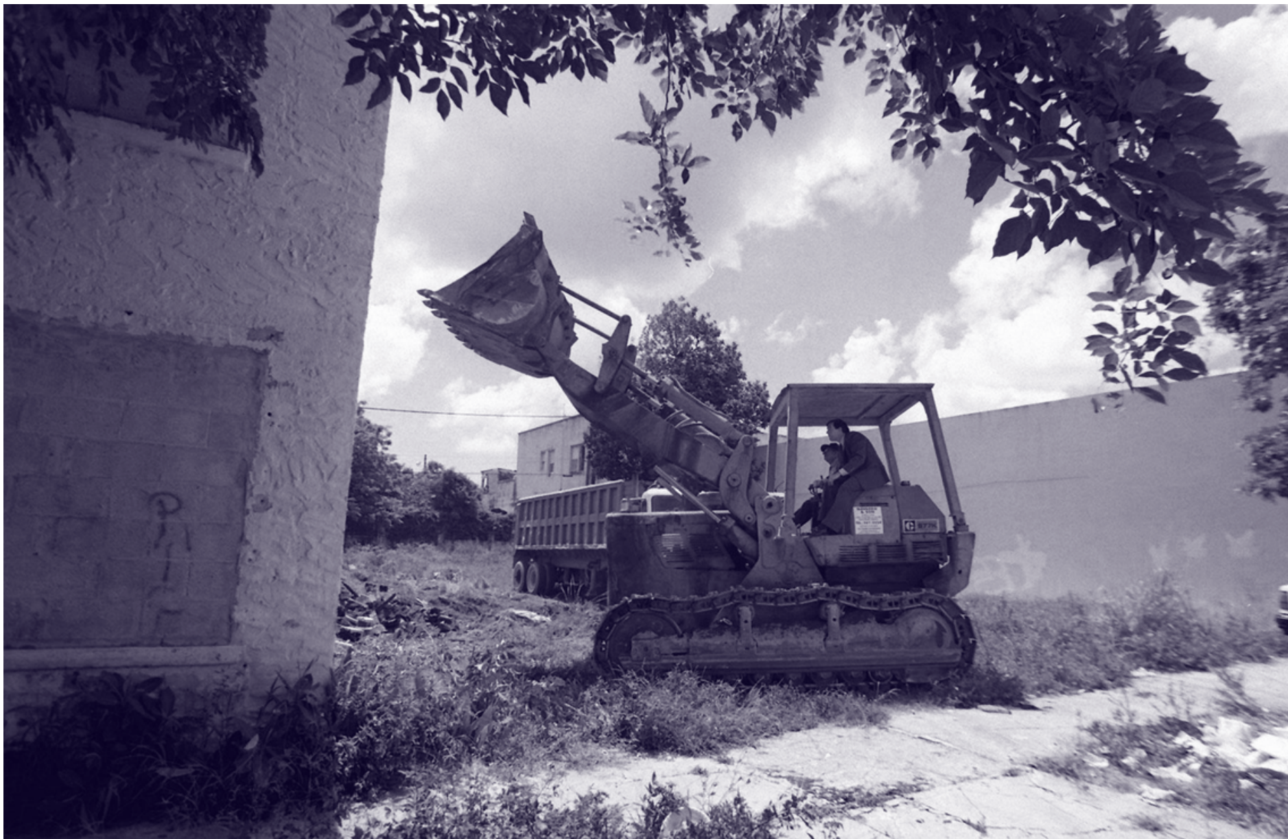
Carollo, then mayor, sits next to the operator of a bulldozer in 1997 as the city tears down an alleged crack house at 1421 NE Miami Ct. A. Enrique Valentin el Nuevo Herald
